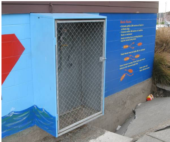
The concrete smashed and the LPG cylinders dropped by approx 450mm.
