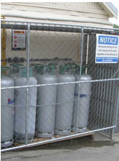
The properly restrained and caged LPG cylinders were unaffected by the earthquake.
