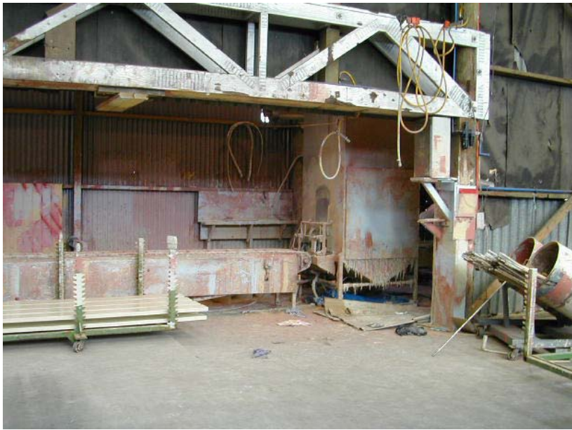
A board spray painting unit, together with the appropriate area classification drawing.
